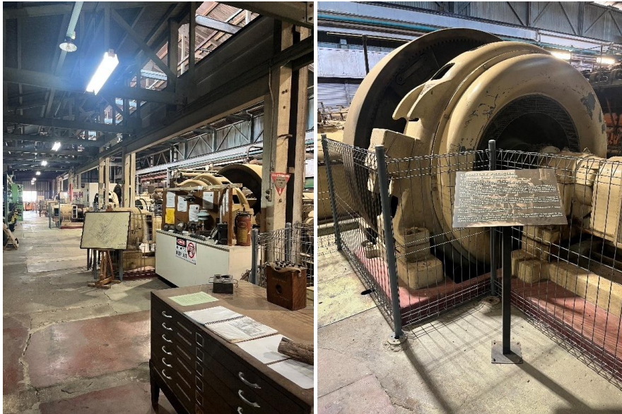
Figures 9 & 10: Powerhouse Generating Complex
